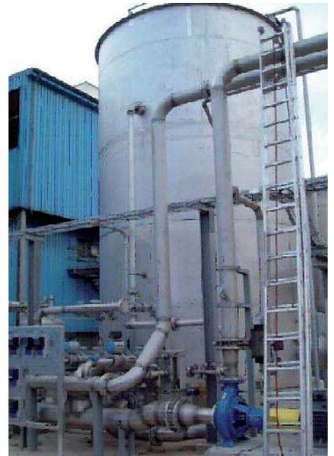
Flotation plant at Schoellershammer paper mill
